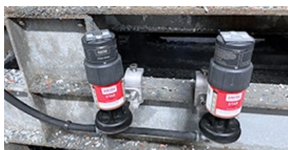
Lubrication of an electric motor on the dryer
