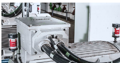
Lubrication of electric motor
