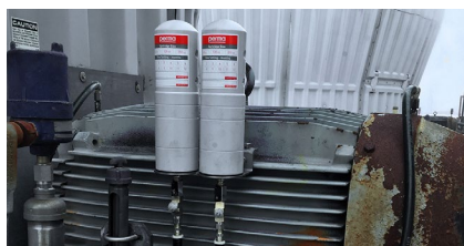
Lubrication of electric motor
