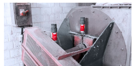
Lubrication of a blower bearing
