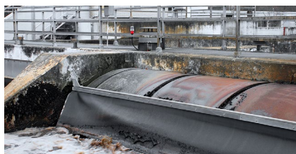
Bearing lubrication at the fan of the aerated tank
