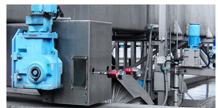
Wheel bearing lubrication at circular scraper
