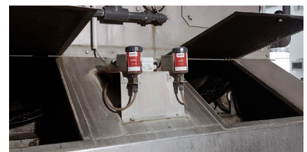
Bearing lubrication at excess sludge densifier
